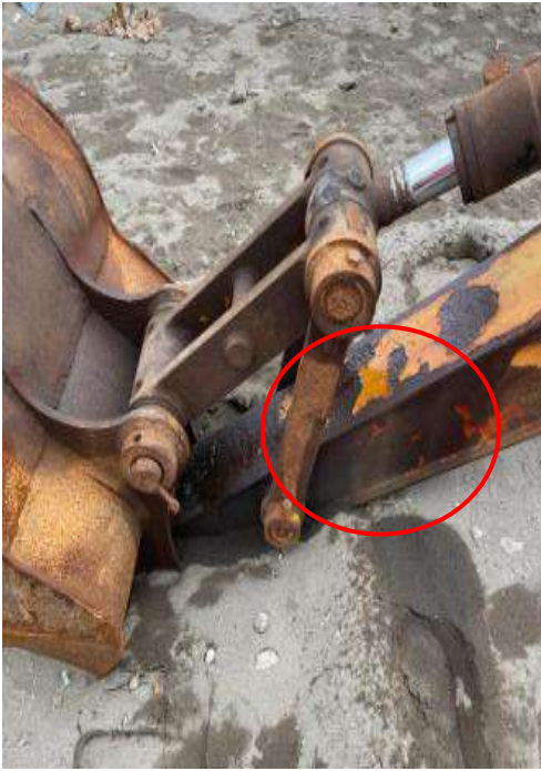
Fig. 4. Condition of the bucket cylinder housing with the hydraulic oil leak.
