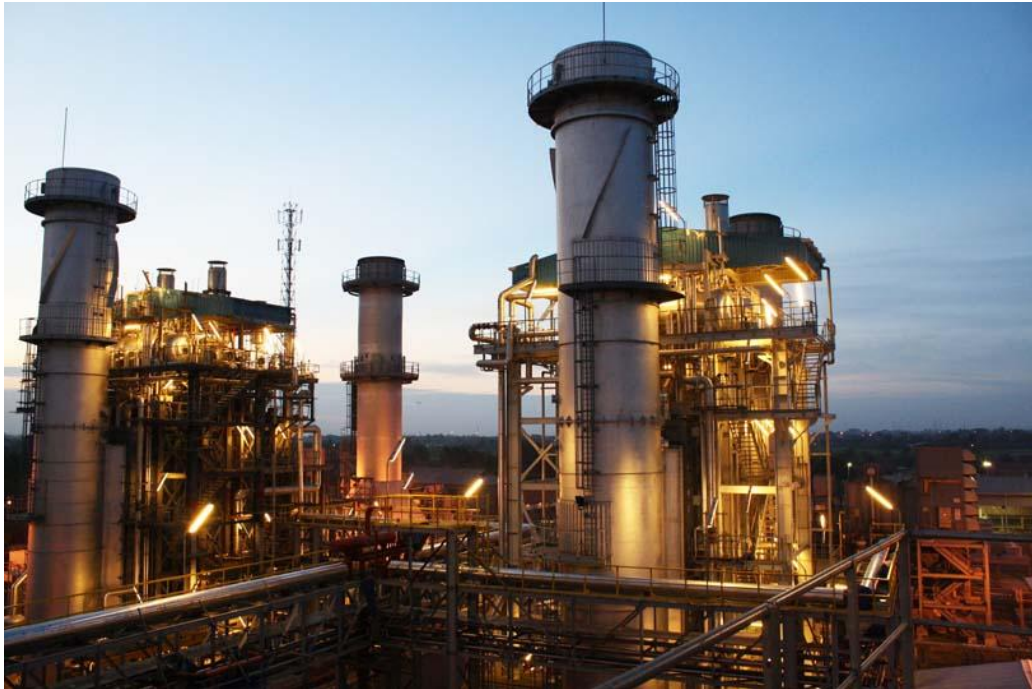
Figure 4.1 PT. Bekasi Power
